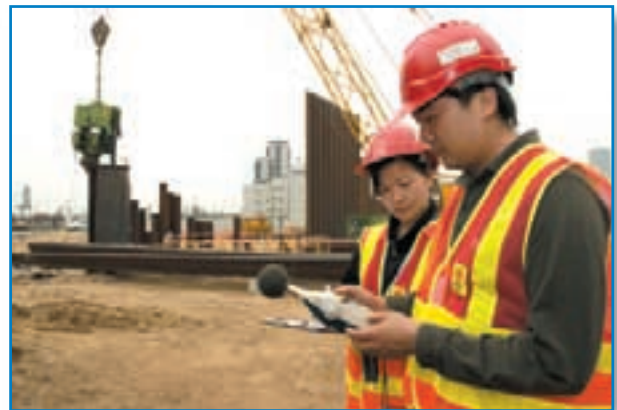
The Group actively participates in maintaining an environmentally friendly construction site to minimize its pollution to the environment.
