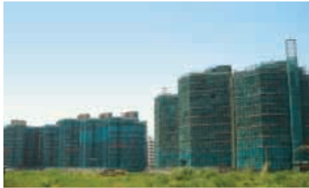
Construction site of Long Dong Cun at Guangshan Road Western, Tianhe District, Guangzhou, Guangdong Province, PRC
