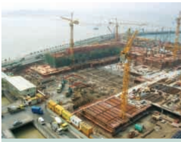
Piling, pile caps and basement construction work at MGM Grand Macau at Nam Van, Macau undertaken by Chinney Timwill Construction (Macau) Co., Ltd.
