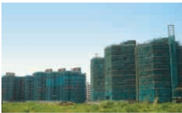
Construction site of Long Dong Cun at Guangshan Road Western, Tianhe District, Guangzhou, Guangdong Province, PRC held by Hon Kwok Land Investment Company, Limited
