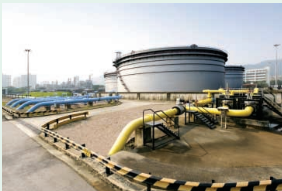
The Tai Po gas plant is currently using dual feedstock mix – naphtha and natural gas, bringing cost savings to customers and helping to protect the environment.
