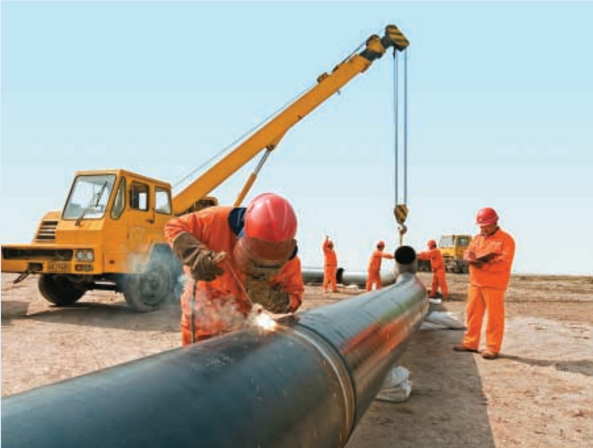
In a joint tri-partnership, Hong Kong and China Gas has participated to construct a high-pressure natural gas pipeline system in Hangzhou that will eventually supply household, commercial and industrial business customers.
