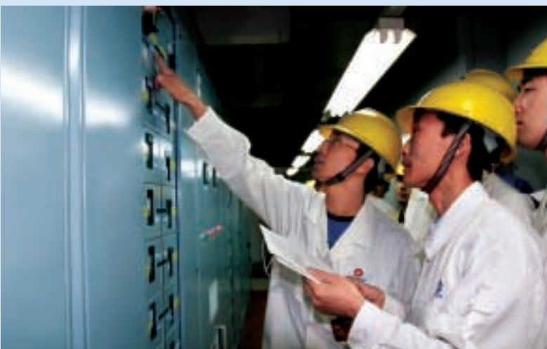
Checking of operating equipment in the power plants
