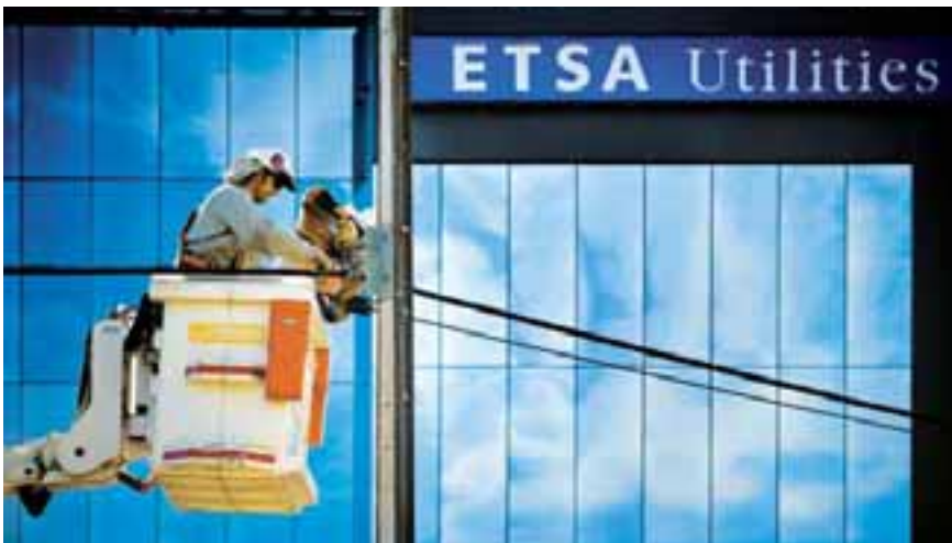
ETSA Utilities is the primary electricity distribution business for the state of South Australia.
