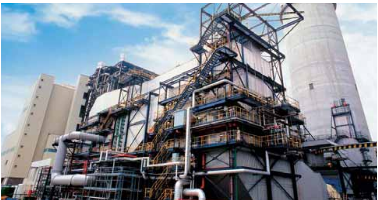
Unit 9, commissioned in October 2006, increases the generating capacity of Lamma Power Station from 3,420 MW to 3,755 MW, as well as helps to reduce emissions through the use of natural gas.
