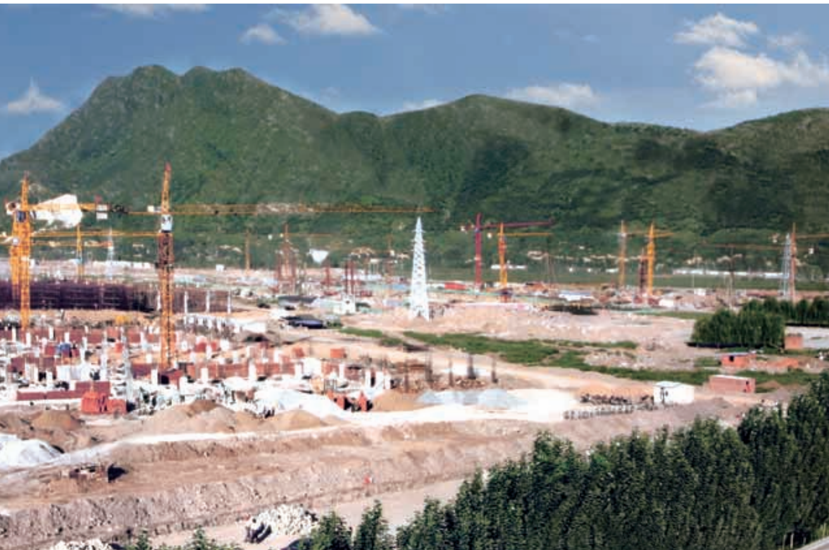
The Group's new plant under construction in Chaoyang, Liaoning Province, the PRC
