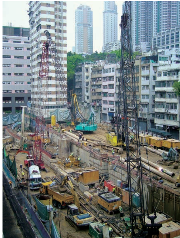
Bored piling works at First Street and Second Street of Sai Ying Pun, Hong Kong undertaken by Kin Wing Engineering Company Limited
