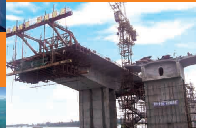
Construction of Phase II of the Western Delta Route linking Shunde to Zhongshan (Under Construction)
