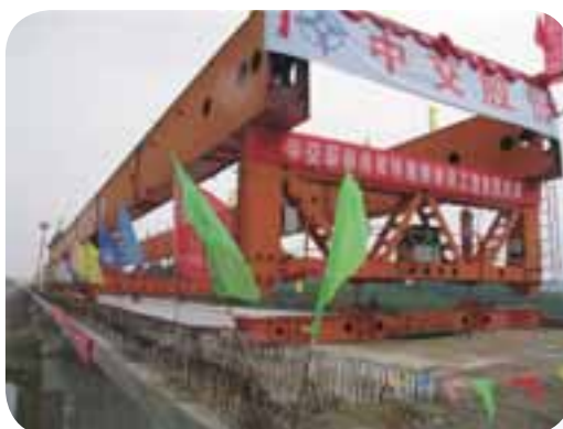
The completion of construction for switch tower box at Hongan Liangchang for Wuhe Railway
