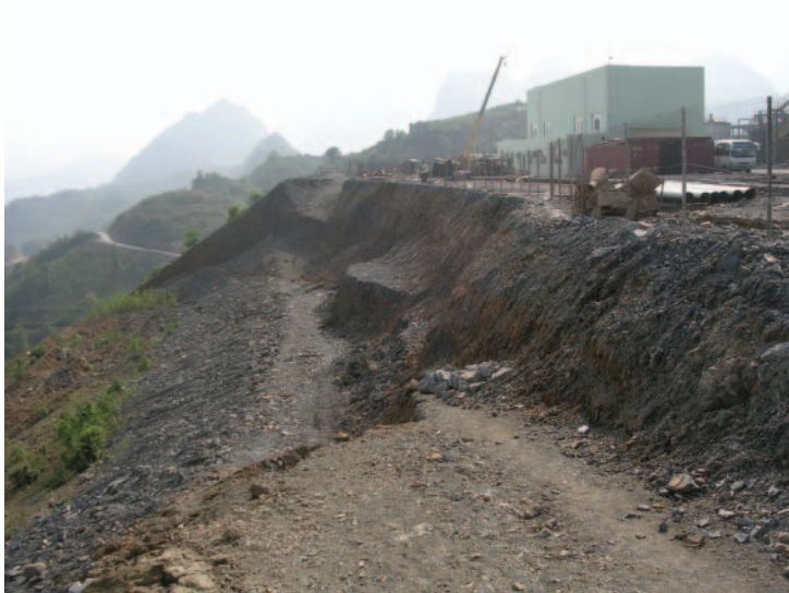
Figure 5-30: Photograph Showing Plant Site Embankment Failure, 15 October 2006
