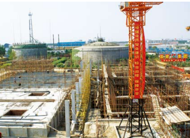
Refurbishment work for Zibo Waste Water Treatment Plant 淄博污水處理廠改造工程
