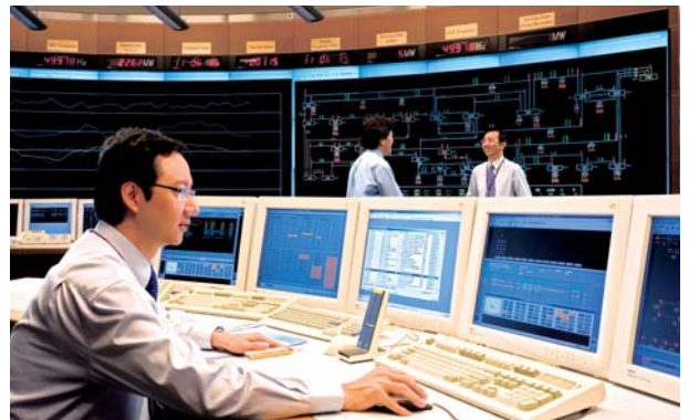
The state-of-the-art supervisory control and data acquisition (SCADA) system helps HK Electric maintain exceptional reliability.
