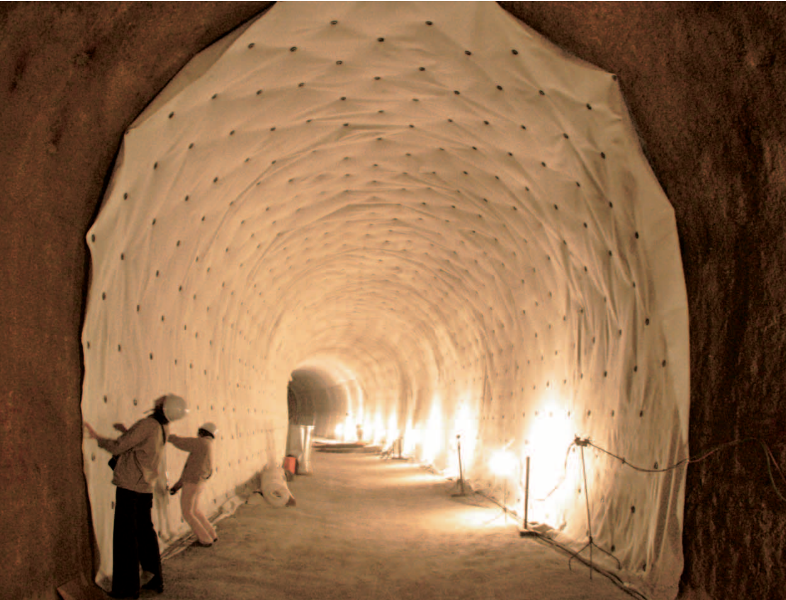
14 stations have been handed over to the B JL4 PPP company to start E&M installation
