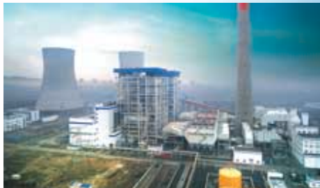
Yaomeng Power Plant II
