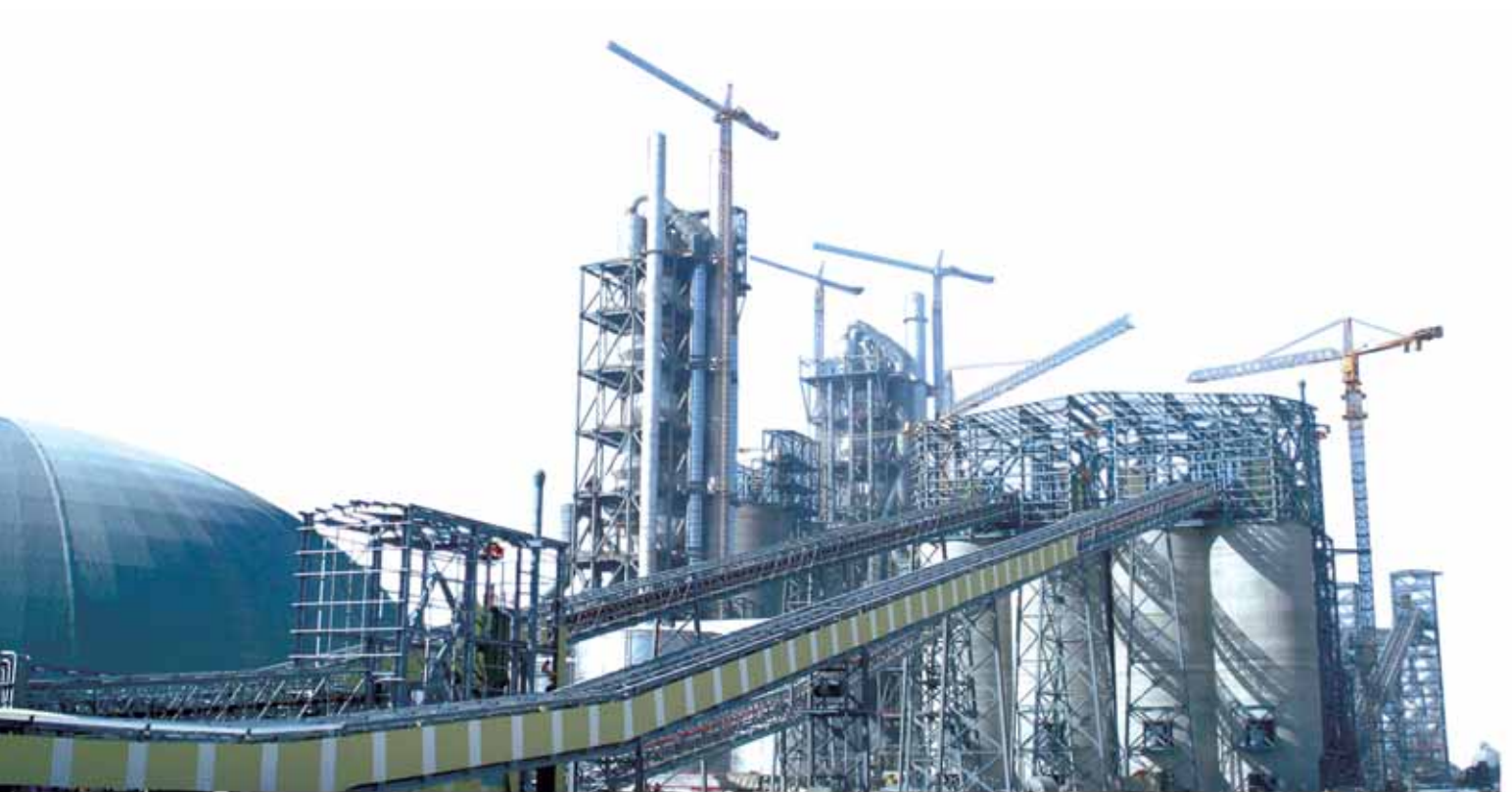
SCC 10,000TPD cement production line, Saudi Arabia
