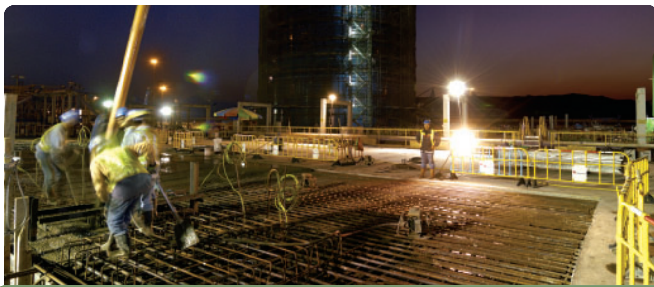
Working around the clock on the Emissions Control Project at Castle Peak “B”
