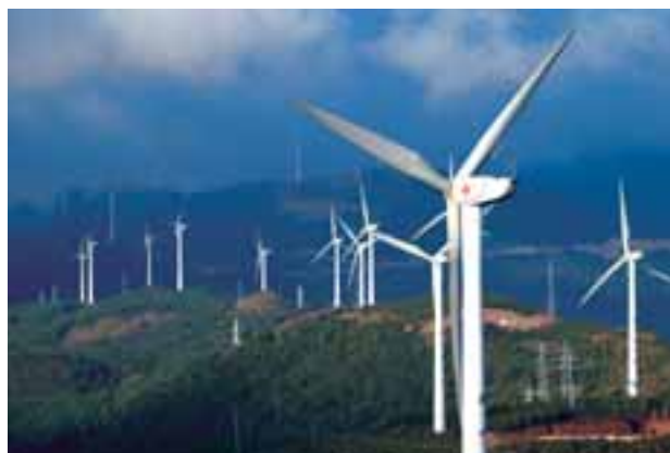
HK Electric's 48 MW wind farm in Dali, China has commenced operations in January 2009.
