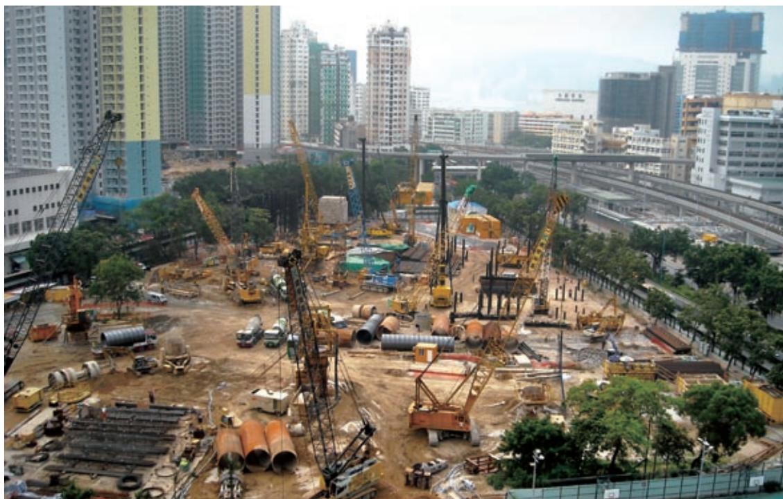
Foundation piling works undertaken by Kin Wing Engineering Co., Ltd., Chinney Alliance Group
