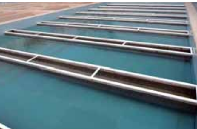
Macau Water Plant
