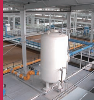
Tianjin Jieyuan Water Plant
