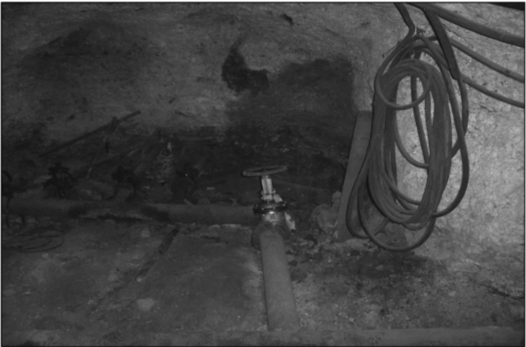
Underground Mirabilite Pipeline System Note Dual Pipeline Discharge Pipes from Production Cell
