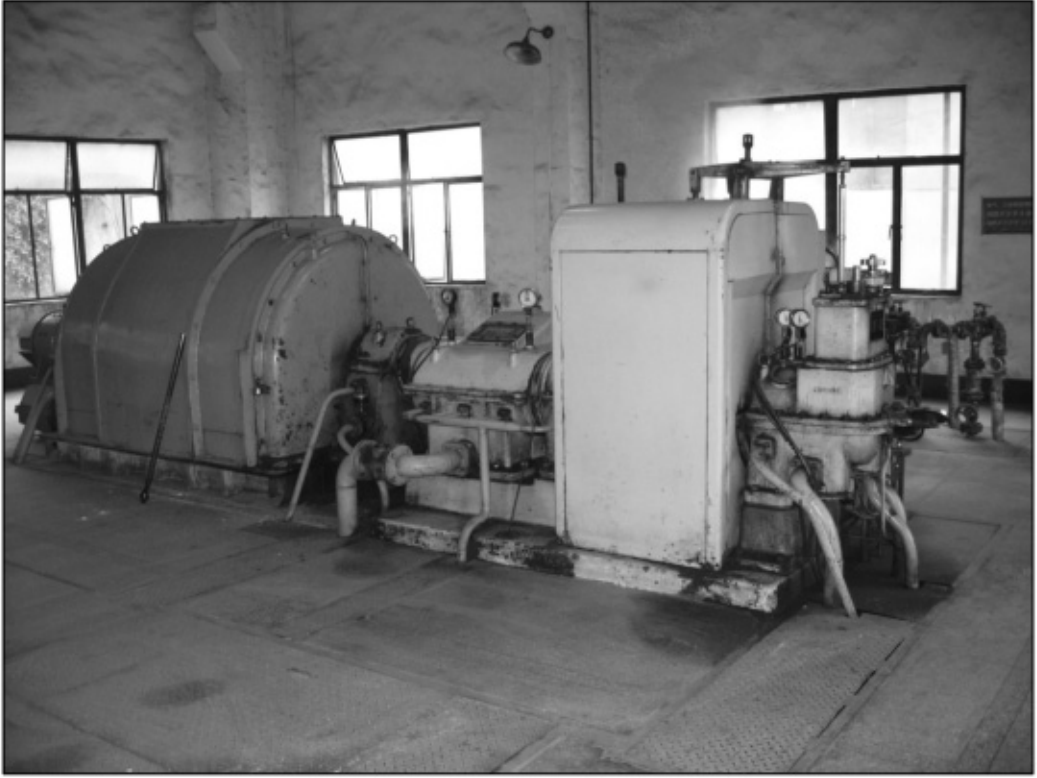
Dahongshan Power Plant Turbine Room
