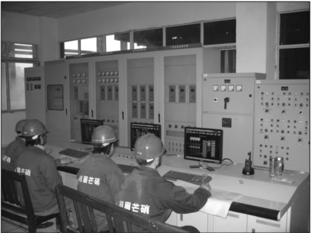
Control Room of Power Plant
