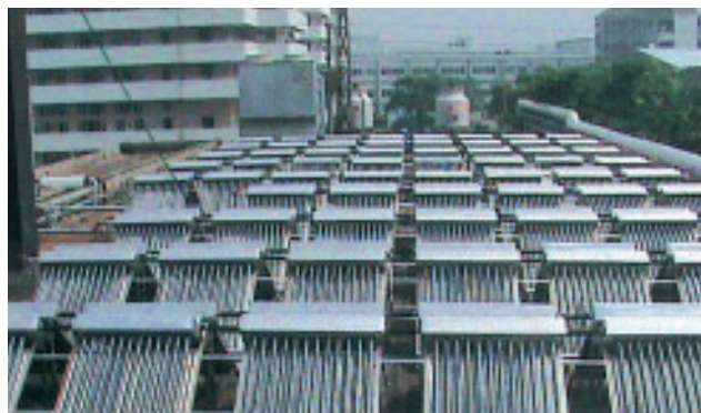
Solar panels at the Prime Asia Leather factory facility enabling natural sunlight to heat the water added in the leather manufacturing process. (Huangjiang Dongguan) 東莞黃江的普愛亞細亞皮革廠房設施的太陽能板，有助利用自然太陽光加熱皮革製造過程中所注入的水。
