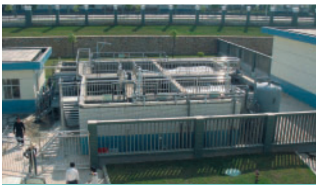
2nd stage completed of the expansion program for the new water treatment facilities for the factory. (ShangGao Jiangxi) 江西上高廠房的新污水處理設施擴展計劃的第二階段竣工。
