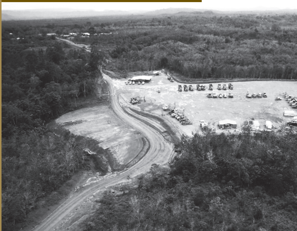
05/ The bulk earthworks at the Martabe Project site 礦地大型土建工程
