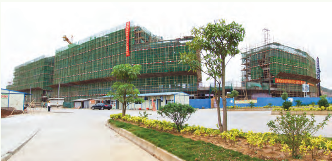
於廣東封開在建中的員工宿舍 Employees' dormitory under construction in Fengkai, Guangdong
