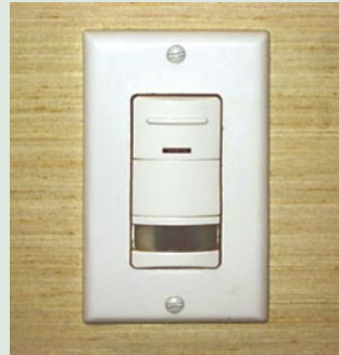
The Peninsula New York installed motion sensors in back of house areas to reduce energy consumption when areas are not in use.
