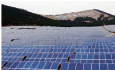
Xuzhou Solar Farm
