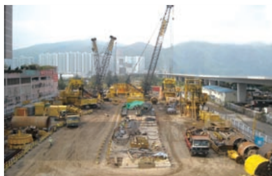
Foundation piling works undertaken by Kin Wing Foundation Limited, Chinney Alliance Group
