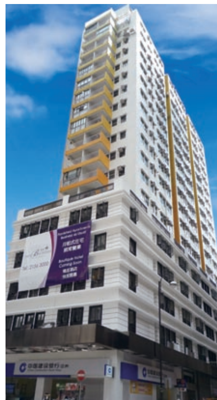
The Bauhinia Hotel (Central) under renovation and The Bauhinia serviced apartments upstairs
