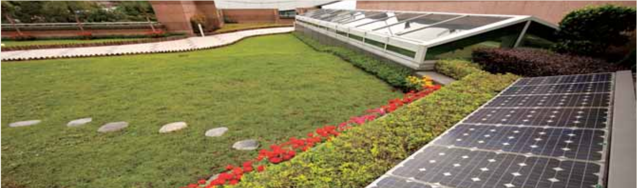
山頂廣場之太陽能發電系統。 The solar panel renewable energy system at The Peak Galleria.
