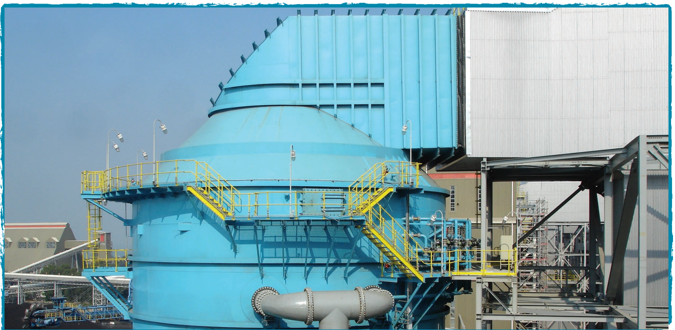
Emissions reduction at Castle Peak Power Station – new Absorber Tower which removes sulphur dioxide from flue gases
