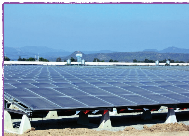
.....to solar farm
