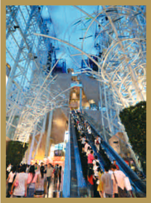
Expressescalators at Langham Place Mall
