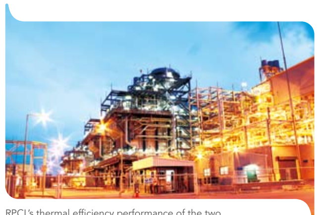
RPCL's thermal efficiency performance of the two combined-cycle gas turbine blocks has exceeded targets.
