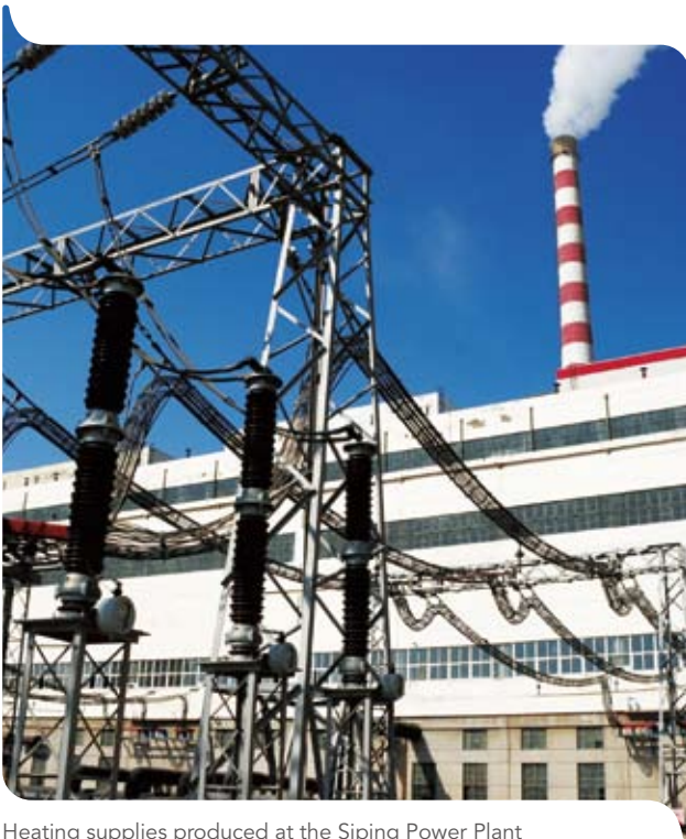
Heating supplies produced at the Siping Power Plant hit a record high in 2010.
