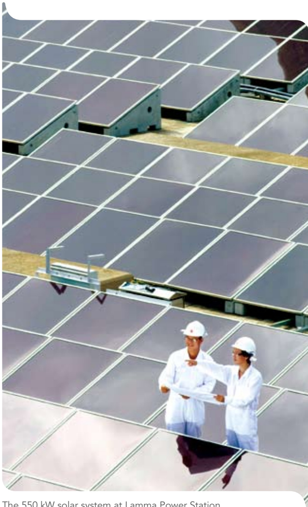
The 550 kW solar system at Lamma Power Station is the largest in Hong Kong.
