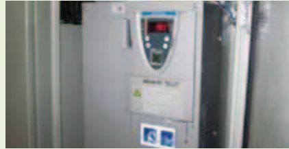
Top : The Peninsula Bangkok's new and more efficient flatwork ironer Above : The Repulse Bay's variable frequency drive unit
