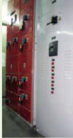
Above : The Repulse Bay's power factor correction equipment
