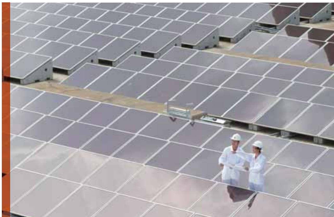
HK Electric commissions Hong Kong's largest solar power system at Lamma Power Station, which comprises 5,500 photovoltaic panels.
