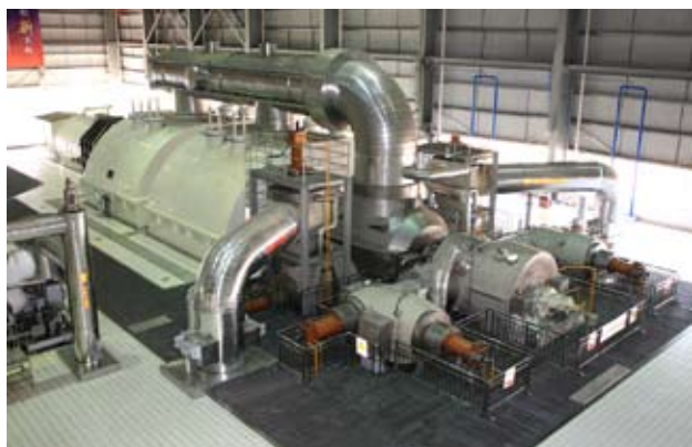
1000MW Ultra Super Critical Power Generation Sets
