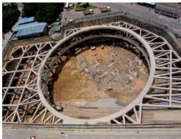
Hon Kwok City Commercial Centre, Futian District, Shenzhen – foundation works in progress
