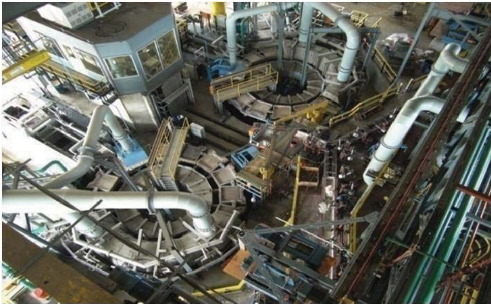
Figure 58: New Twin Anode Casting Wheel (80 tph capacity)
