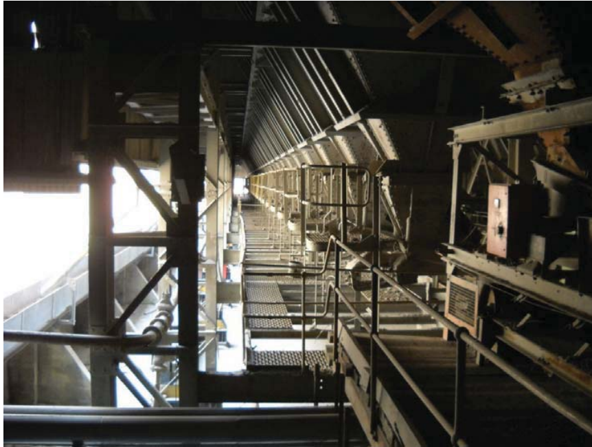
Figure 50: Mill Feed Bin
