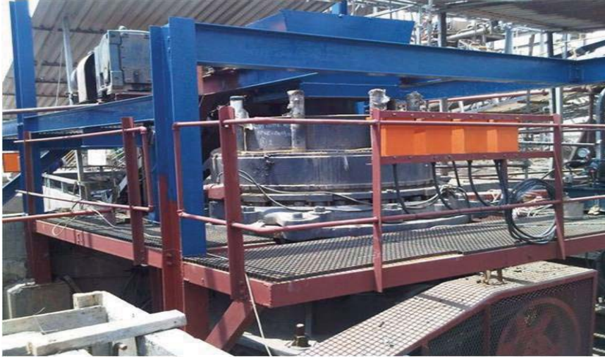
Figure 41: New Standard Crusher in Nkana Leach Plant
