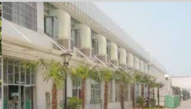
10. A new environmentally friendly ventilation system that reduces the air temperature by 20% 可降低氣溫20%的新環保通風系統
