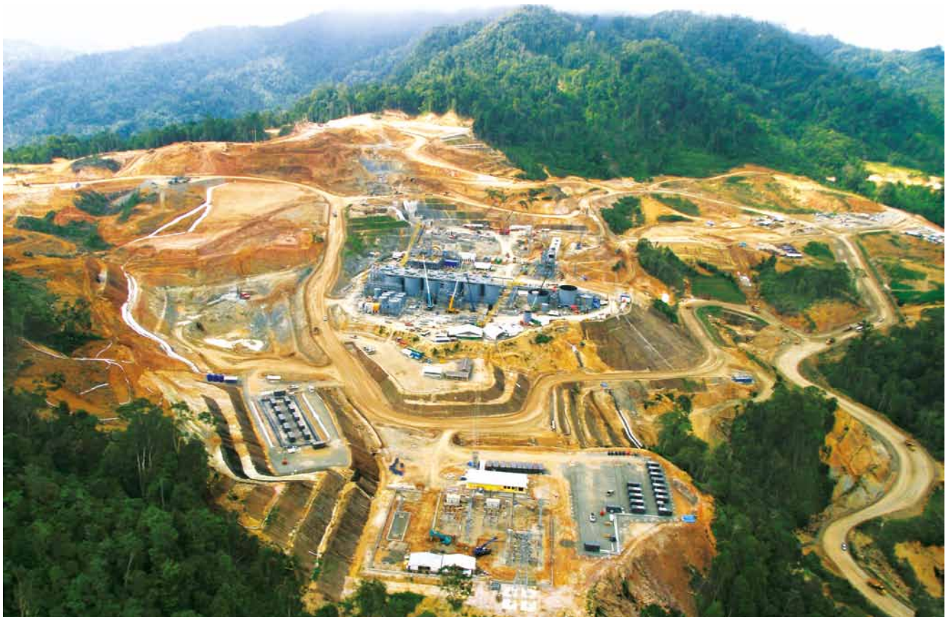
Aerial record of processing plant, high voltage switchyard and fuel area – taken 22 February 2012.
