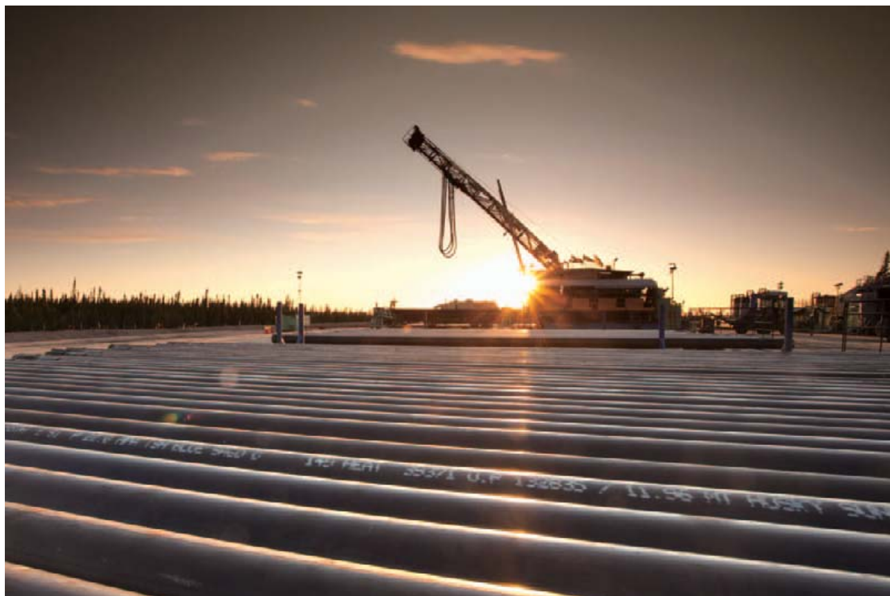
Husky Energy's Sunrise Energy Project in Northern Alberta commences construction on the infrastructure components. Drilling is advanced on the steam assisted gravity drainage horizontal well pairs.
