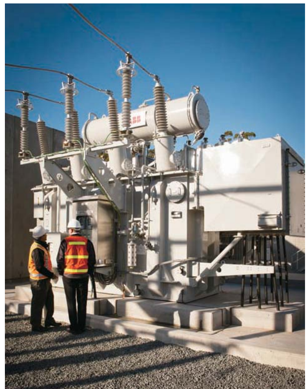
Powercor is Victoria's largest electricity distributor.
