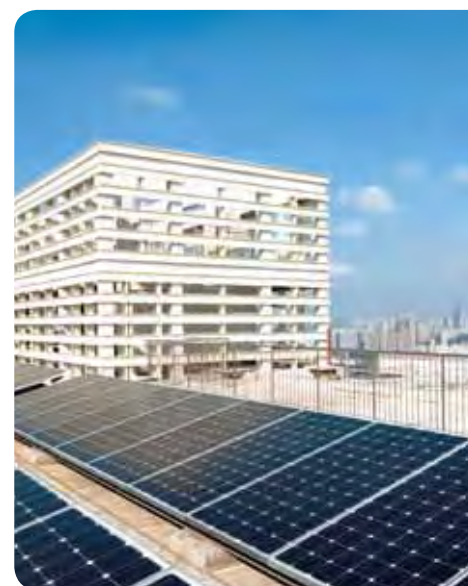
Installed energy-saving solar panels
