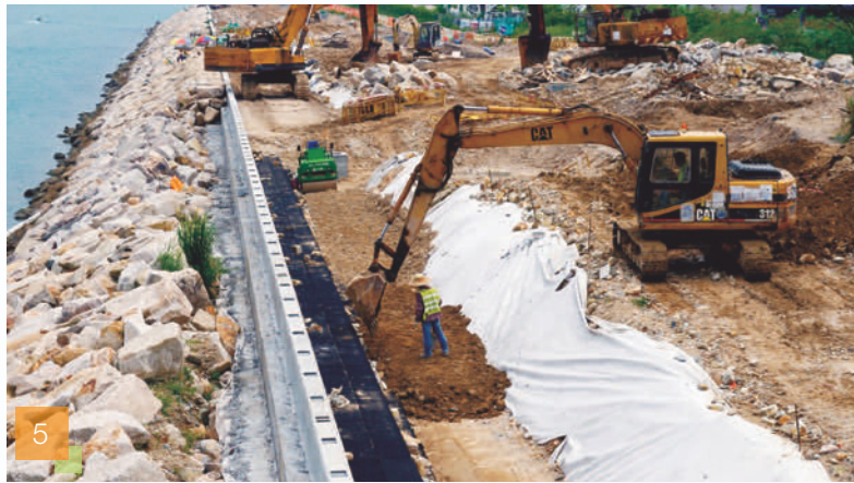
3 Infrastructure Works at Town Centre South and Tiu Keng Leng, Tseung Kwan O 5 Cycle Tracks and Associated Facilities along the Seafront at Tseung Kwan O Town Center South
