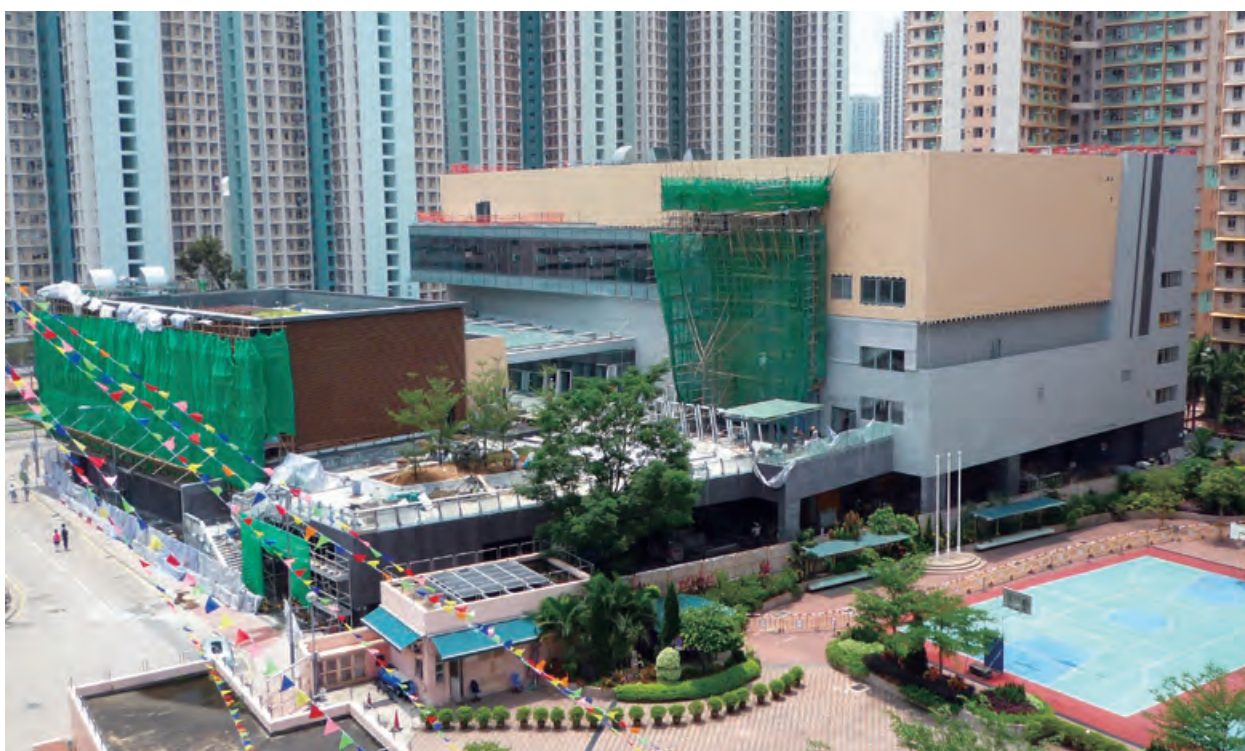
Construction of Sports Centre and Community Hall in Area 101 at Tin Shui Wai with a joint venture partner 與聯營夥伴興建天水圍101區的體育中心及社區會堂
