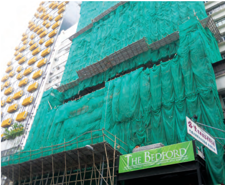
Construction of proposed industrial redevelopment, The Bedford, at No. 93 Bedford Road, Tai Kok Tsui 興建大角咀必發道93號的建議工業重建項目The Bedford
