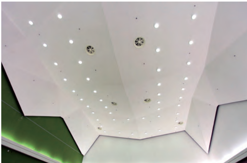
Lam Tin North Municipal Services Building – False ceiling 藍田北市政大樓—假天花系統
