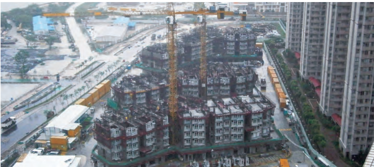
Construction of public rental housing development at Tseung Kwan O Area 65B 興建將軍澳65B區的出租公屋發展項目
