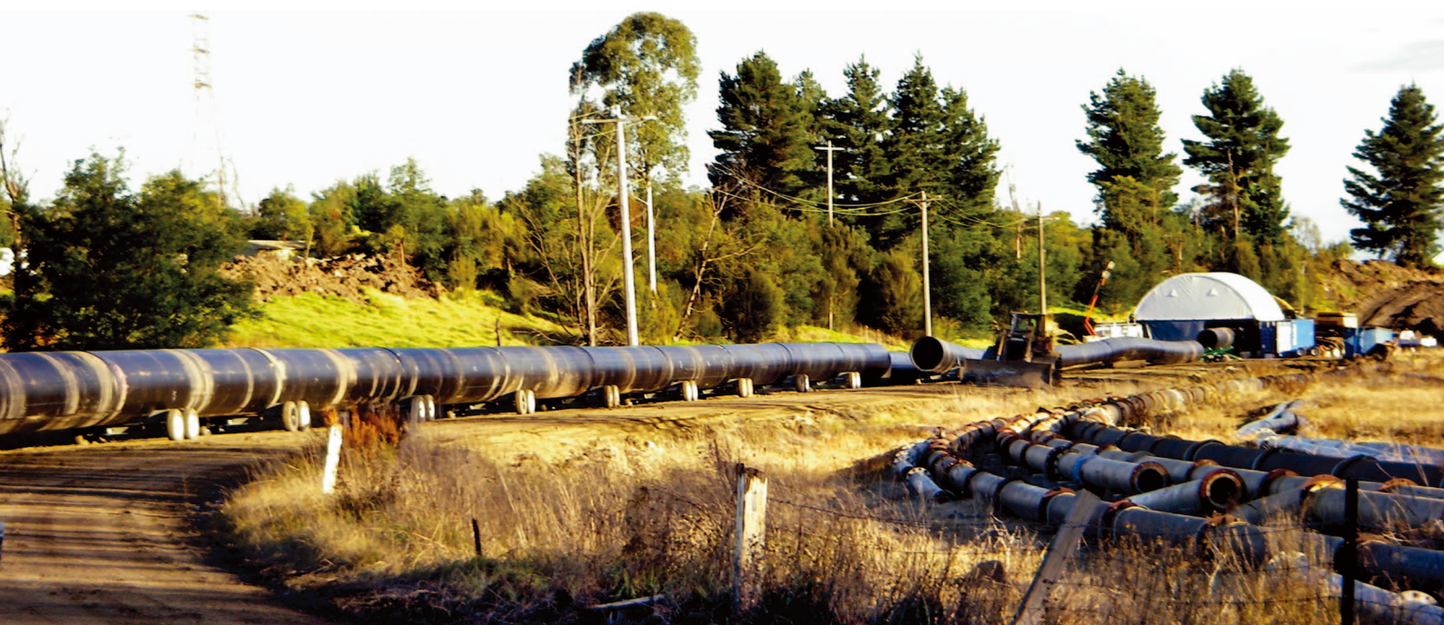
Piping to manage flows of Morwell River across Yallourn coal mine
