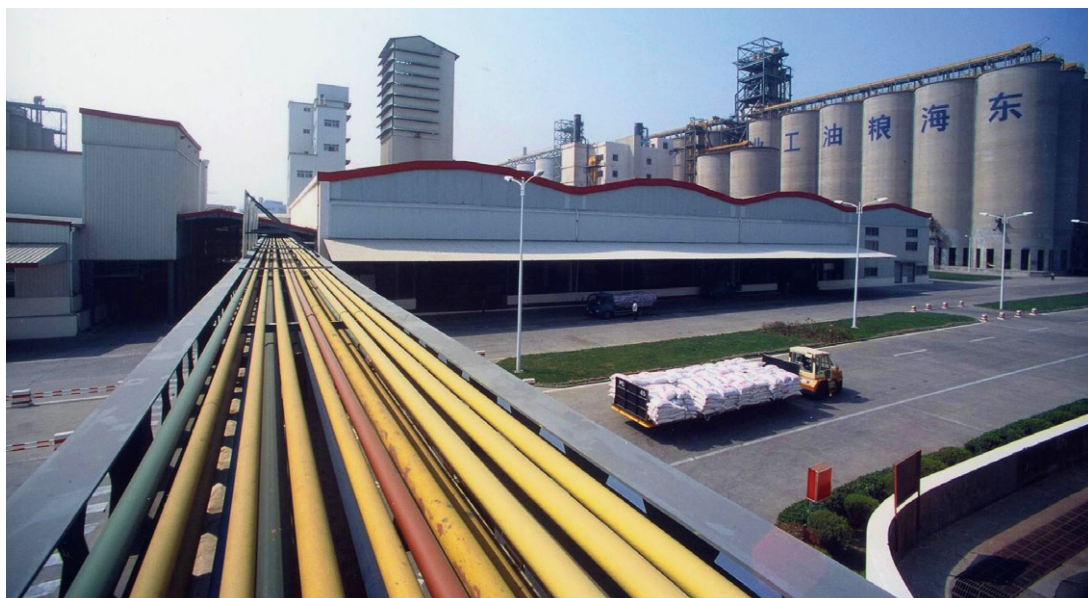
Oil pipelines of COFCO East Ocean Oils & Grains
