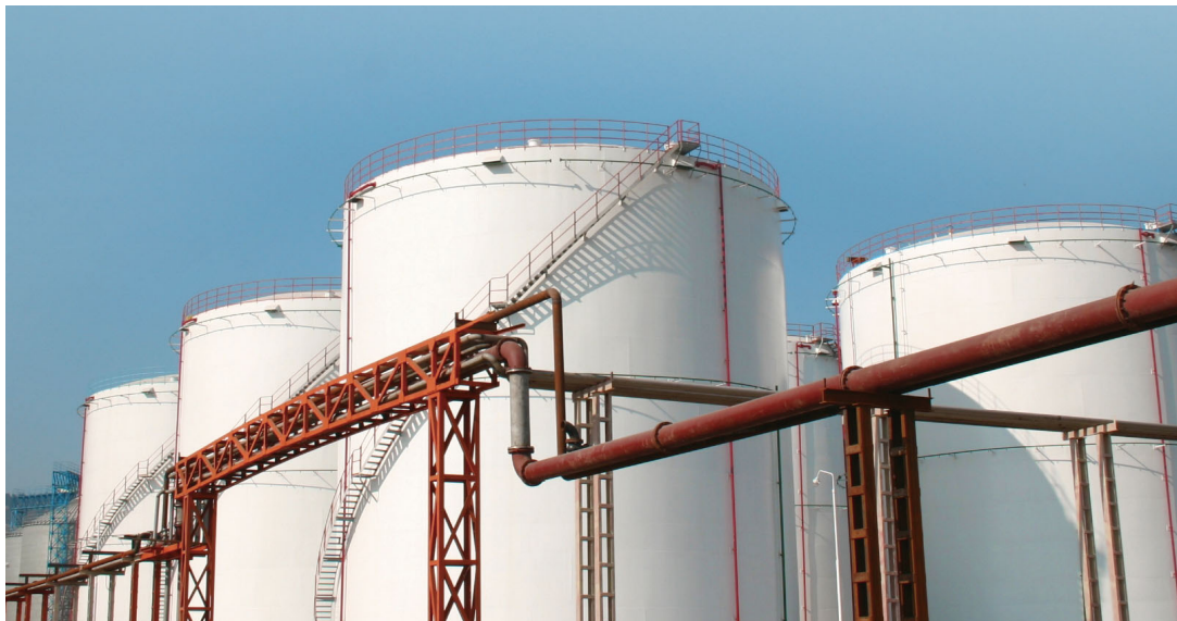
Alcohol storage tanks
