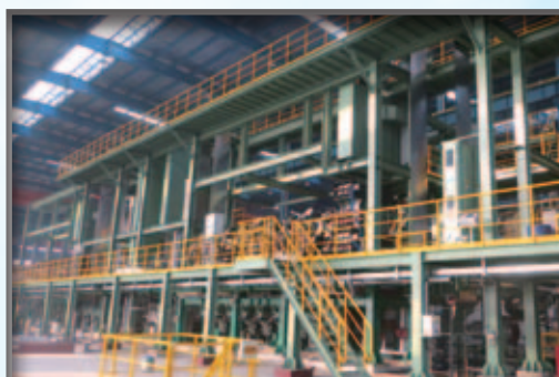
Tinning Production Line
