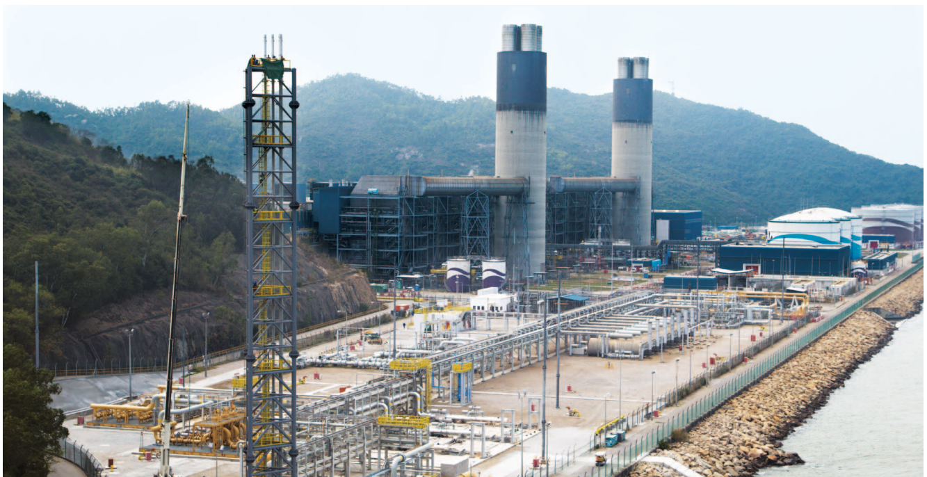
Gas Receiving Station at Black Point
