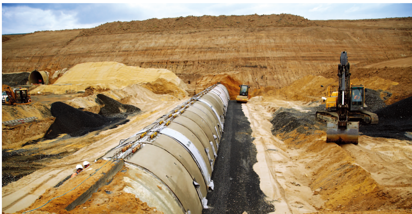
Remediation at Yallourn – restoring a coal conveyor tunnel and rebuilding the river diversion embankment
